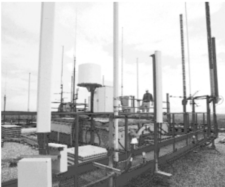
Typical rooftop transmission site. Multiple emitters complicate the measurement process.
